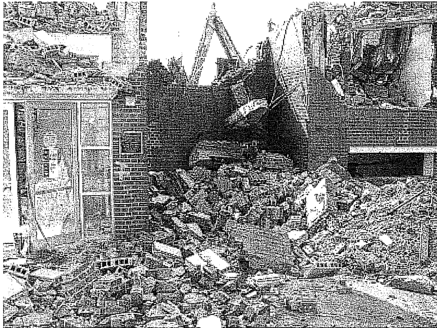
Figure 1.2 A 1960s era student residence hall at the University of Florida in the process of demolition. Although 12,000 bricks were recovered for reuse in new construction, in excess of 90% of the brick was unrecoverable because of the high-strength Portland cement mortar used to bind the bricks together and the lack of provision for disassembly of multistorey brick structures.
